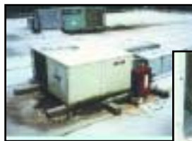
Typical rooftop application with rusted basepan
